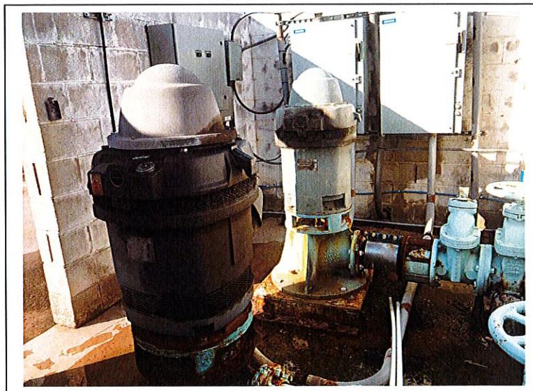
High Service Pump Station on Tower Road
