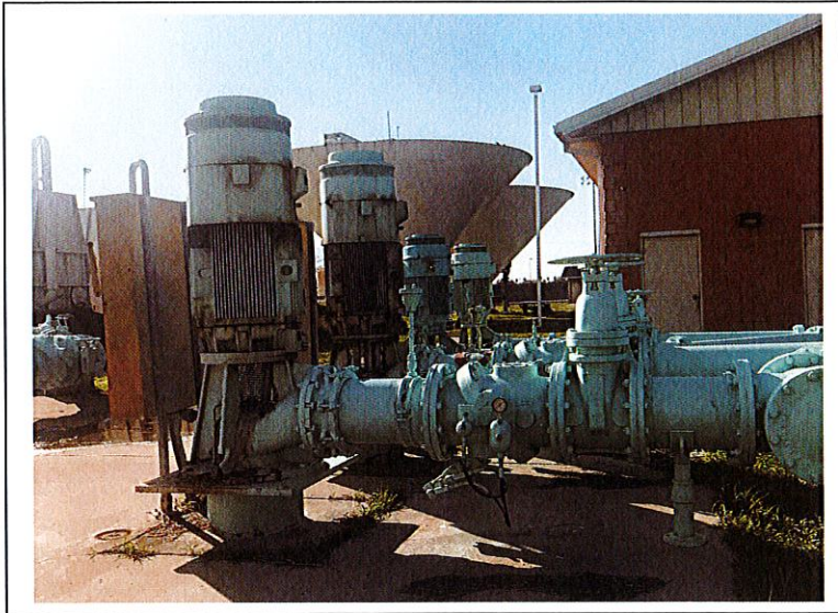
High Service Pump Station- Water Treatment Plant
